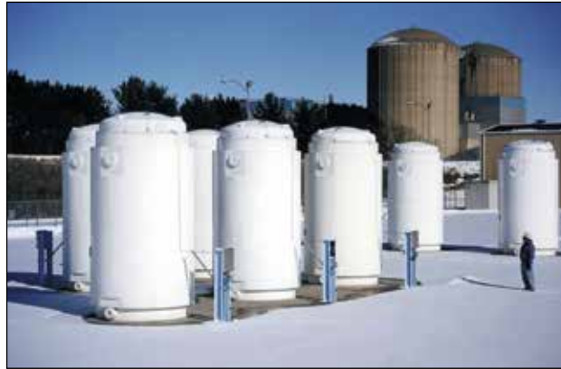
TN-40 Dry Storage Cask
